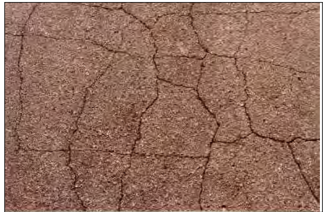
Condition 5 – Very Poor
