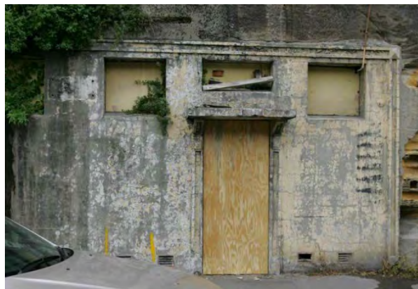
Condition 5 – Very Poor
